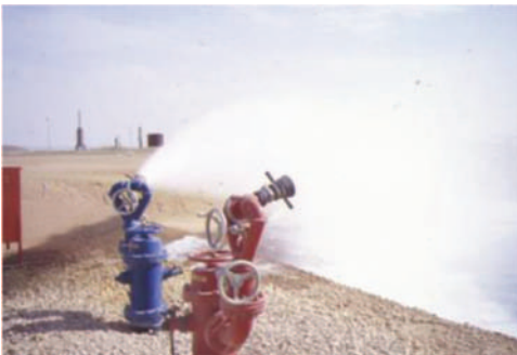
Fixed water monitors will need manual intervention to direct water streams to be fully effective in covering a large and/or wide area. (Picture courtesy Resource Protection International.)
