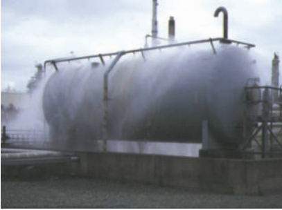
Water spray system in operation. Remote actuation is often necessary to ensure safe operating of the system. (Picture courtesy Resource Protection International.)
