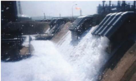
Example of high-expansion foam pourer system into LNG tank bund. (Photo courtesy Angus Fire.)
